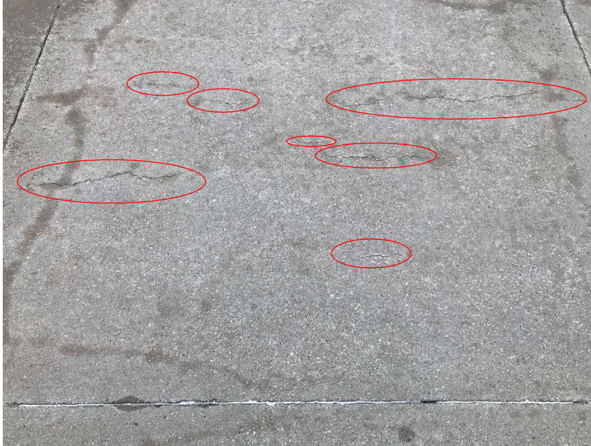
Figure 1-1- Early-age shrinkage cracking in a concrete pavement
